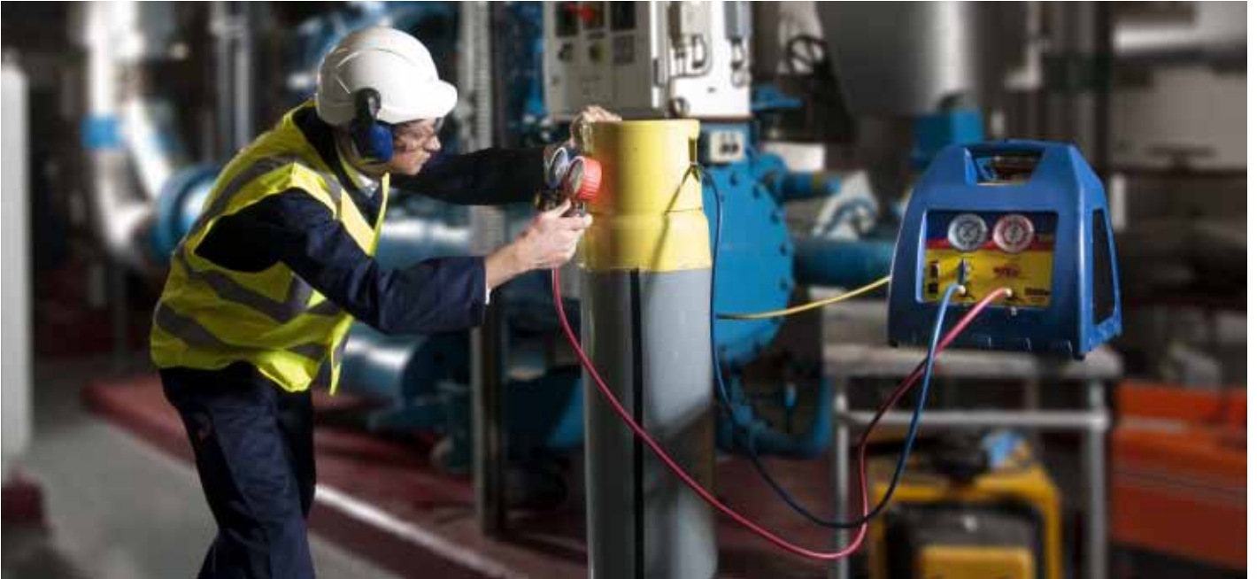
The updated f-gas regulation will impact the use of HFCs in many applications.
